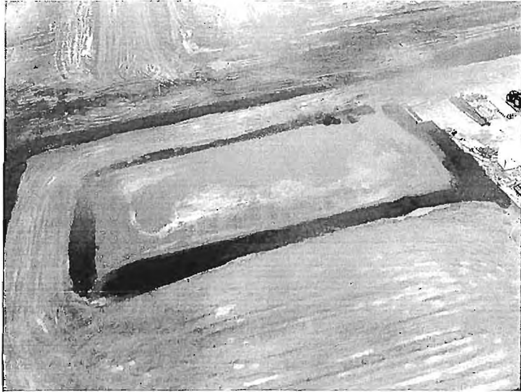
Figure 4 Photograph of the silage leachate containment pond taken on March 7, 2009 before a rainfall event
